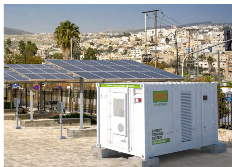
EV Charging Solar + BESS
