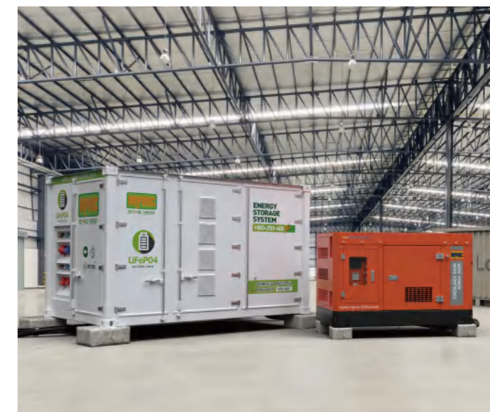
Power Bank & DG
